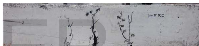
Fig.8 Crack Pattern of HFRC Beams
