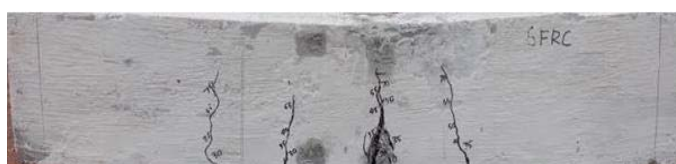
Fig. 7 Crack Pattern of SFRC Beams
