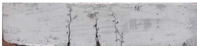
Fig. 5 Crack Pattern of NC Beams
